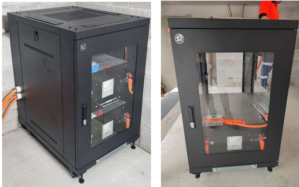
Fig 3. A typical prewired cabinet
